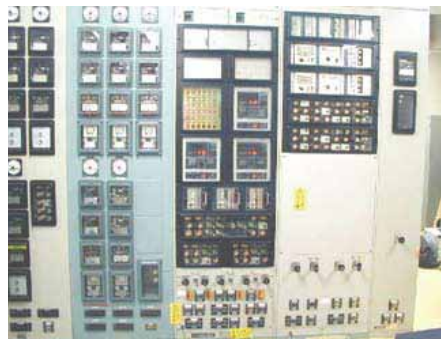
Protective relay devices in generating / transmission substation
