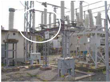
Breakers mounted indoor / outdoor
